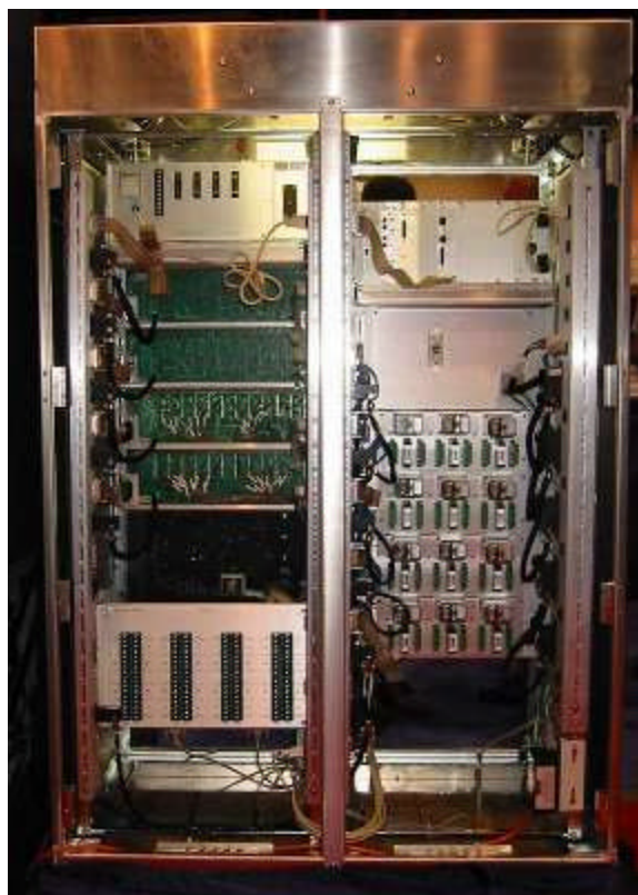
Figure 2: Loose wires are conspicuously absent in this rear view of the new ATC cabinet.
